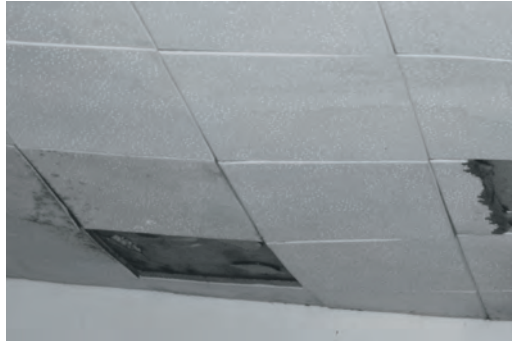
Ceiling tiles that have fallen off due to water damage.
