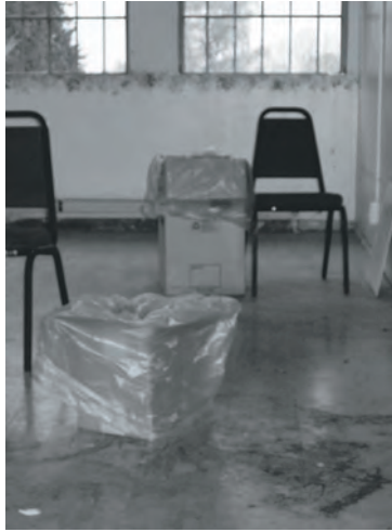
Plastic-lined boxes catching water from leaks.
